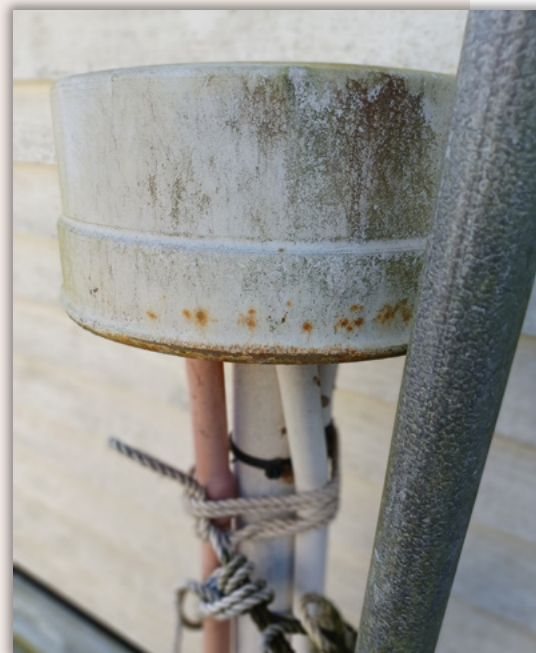
Examples of old and rusty electricity infrastructure in a Residential Land Lease Community.
